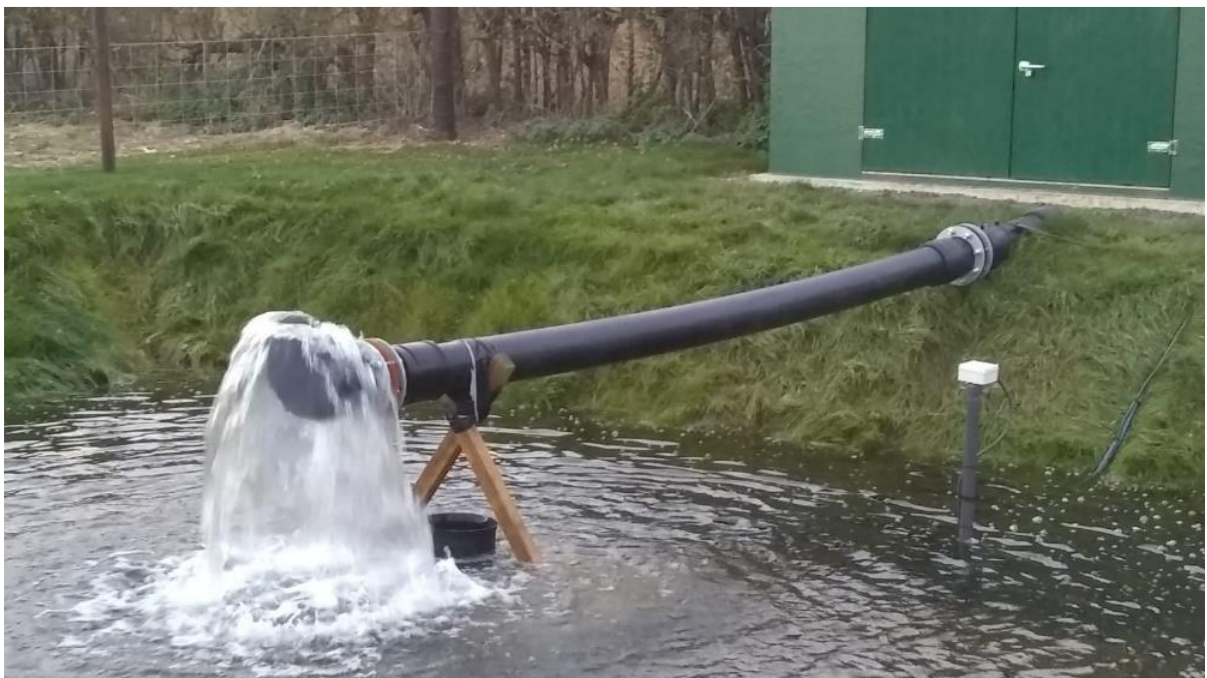
Figure 5. Photograph of recharge lagoon in operation
