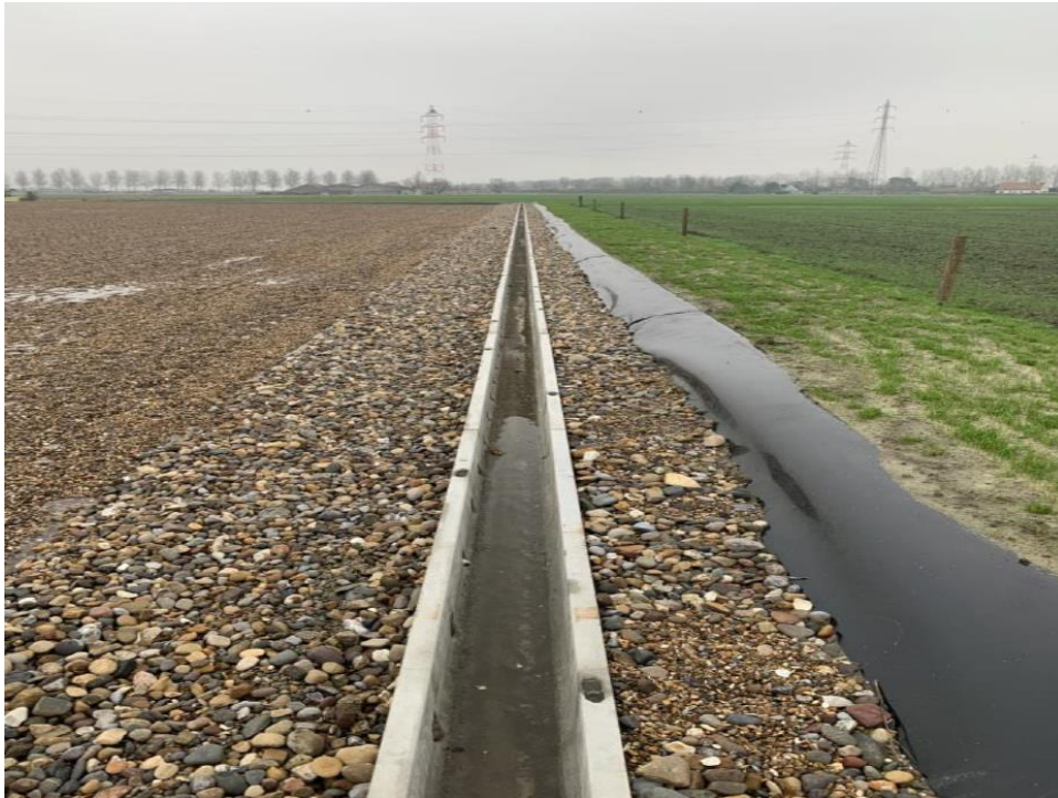
Photo 2. The distribution duct at the south side of the willow marsh
